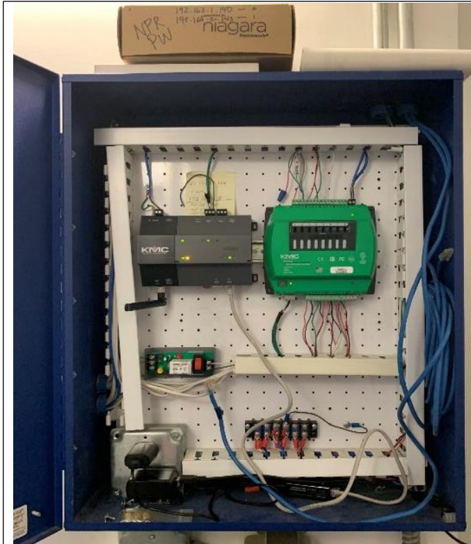
Figure 1 – Controls Panel (KMC Niagara and BACnet)
