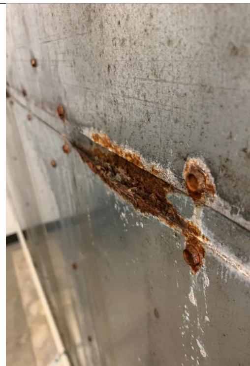
Figure 4 – AHU-2 Bubbling Rust
