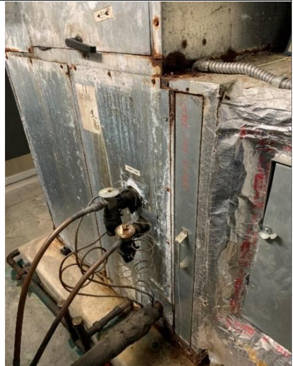
Figure 2 – AHU-2 Liquid and Suction Lines, and Coil Access
