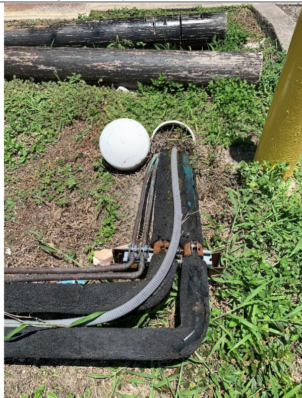
Figure 6 - CU-2 Liquid Line to AHU-2
