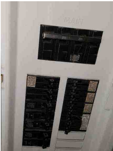
Breaker box in laundry room
