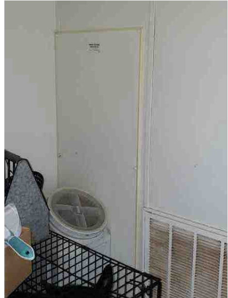
Placement of water heater in laundry room
