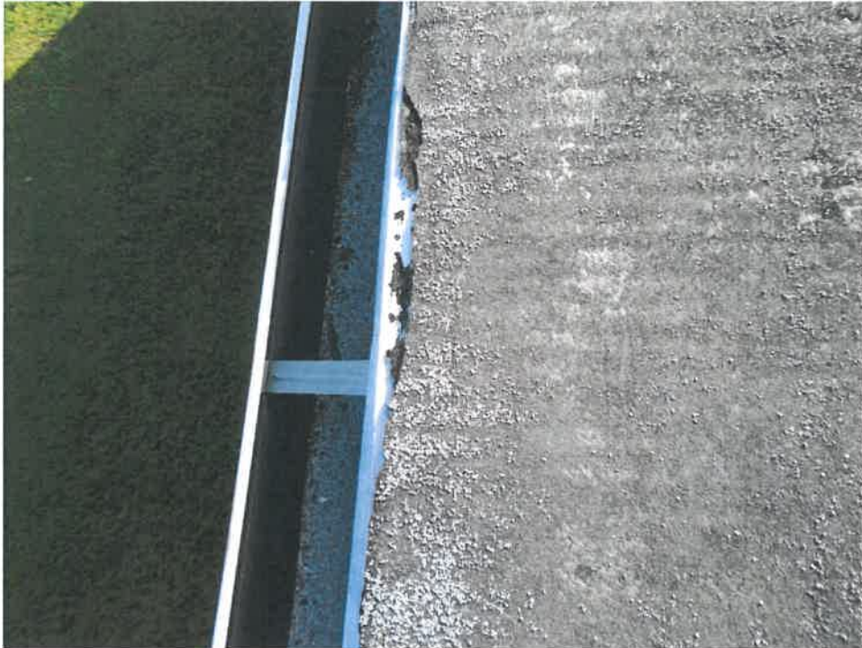
Figure 9: Torn and deteriorated membrane reveals portion of the drip edge around the perimeter of the roof.
