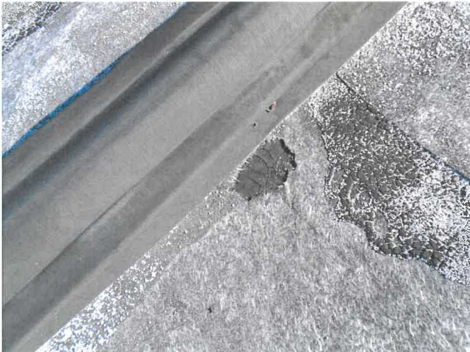
Figure 14: Small areas of deteriorated membrane are visible near the expansion joint.
