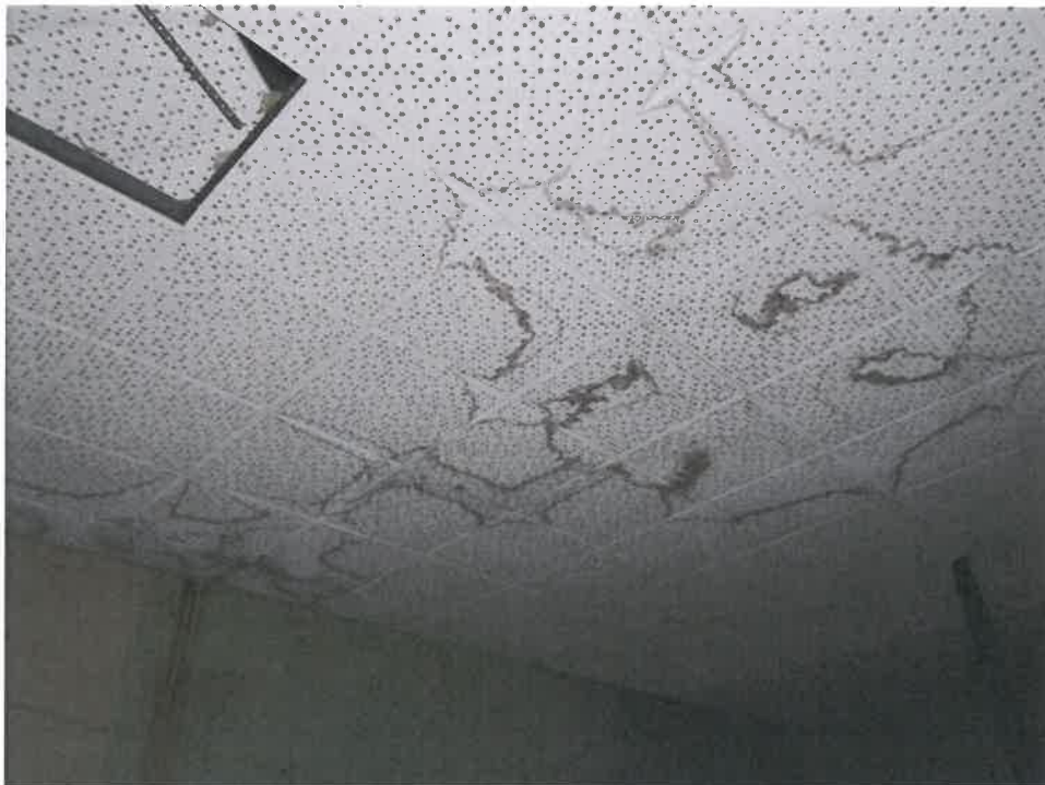
Figure 2: Stains on the original ceiling are visible in a hallway under the north section of roof.
