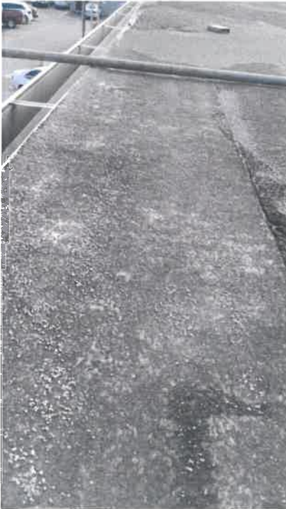
Figure 8: A small depression extends around the perimeter of the north section of roof.
