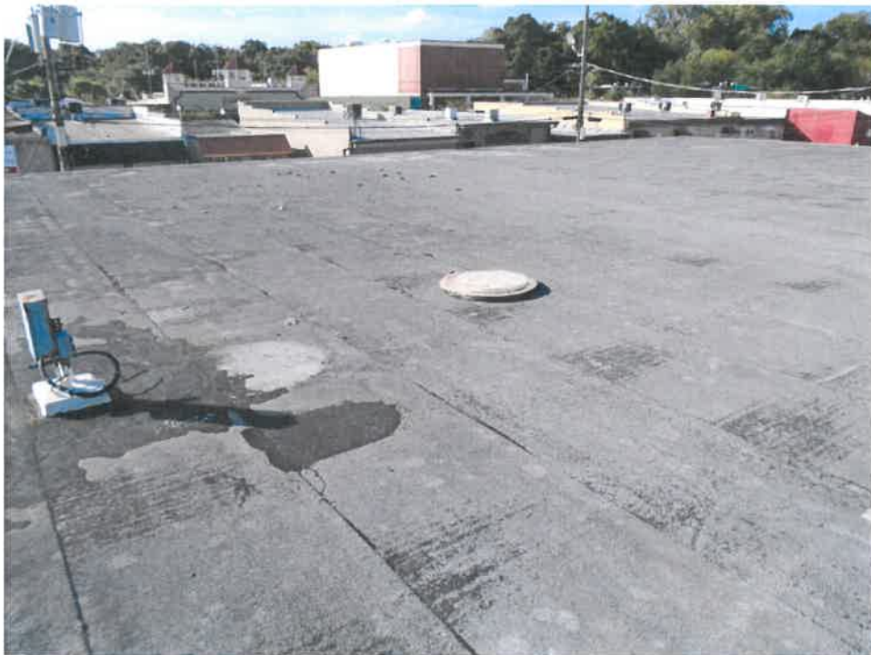
Figure 12: A concrete "disc", chunks of concrete, and sealant around an electrical utility box are visible on the south section of roof.
