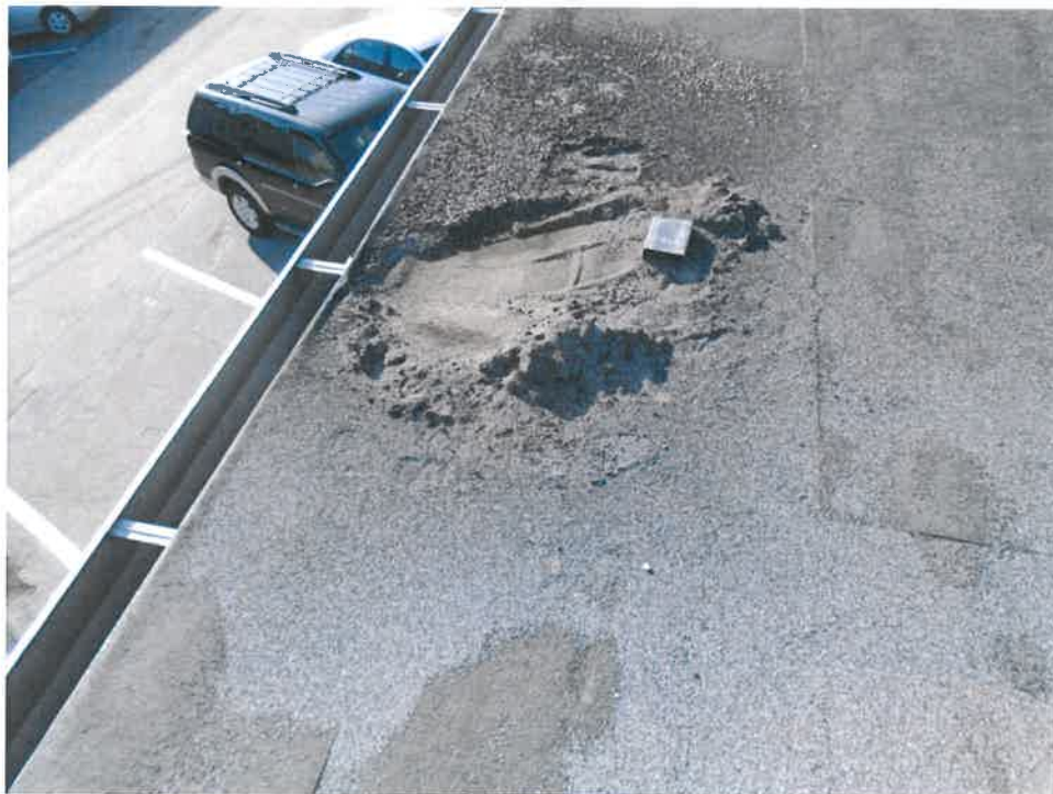
Figure 4: Depressed area in north section of roof where granules have accumulated over 1" thick.
