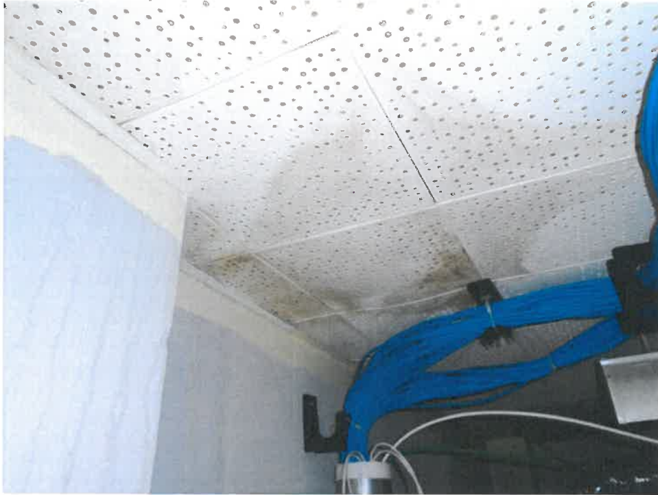
Figure 1: Stains are visible on the original ceiling in a utility room under the north section of roof along the east wall of the building.
