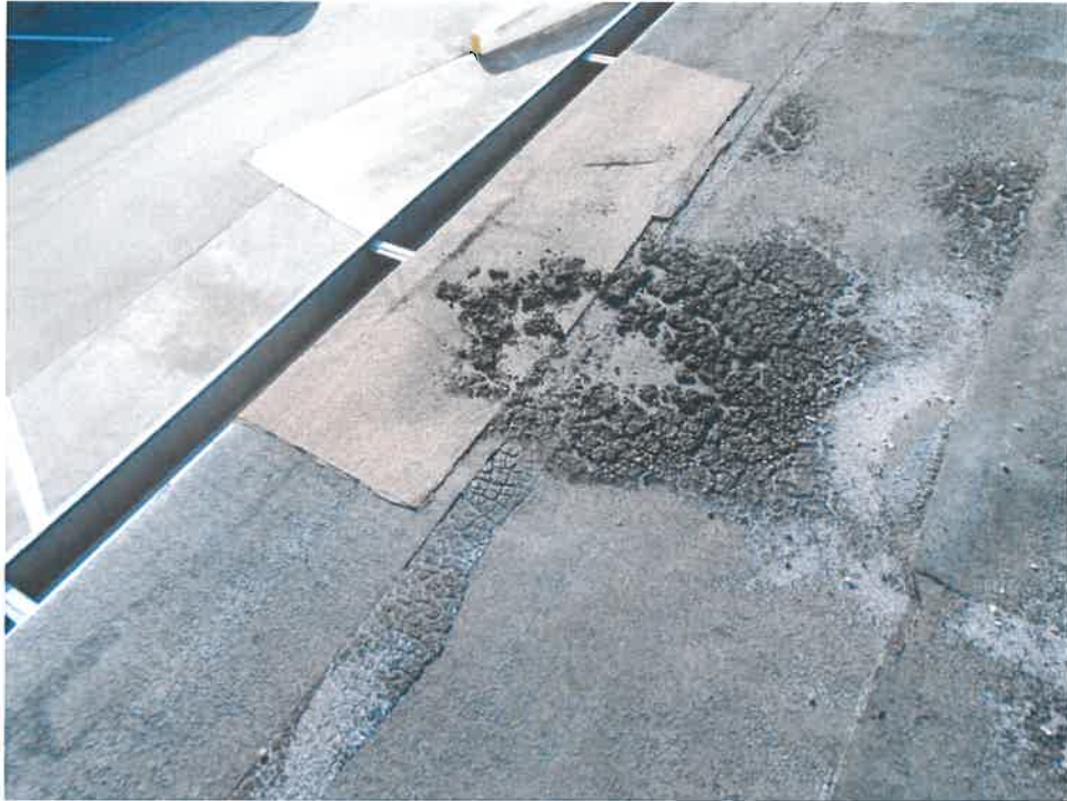
Figure 5: New patch, loose granules, and deteriorated sealant are found over the utility room where water was leaking from the ceiling.
