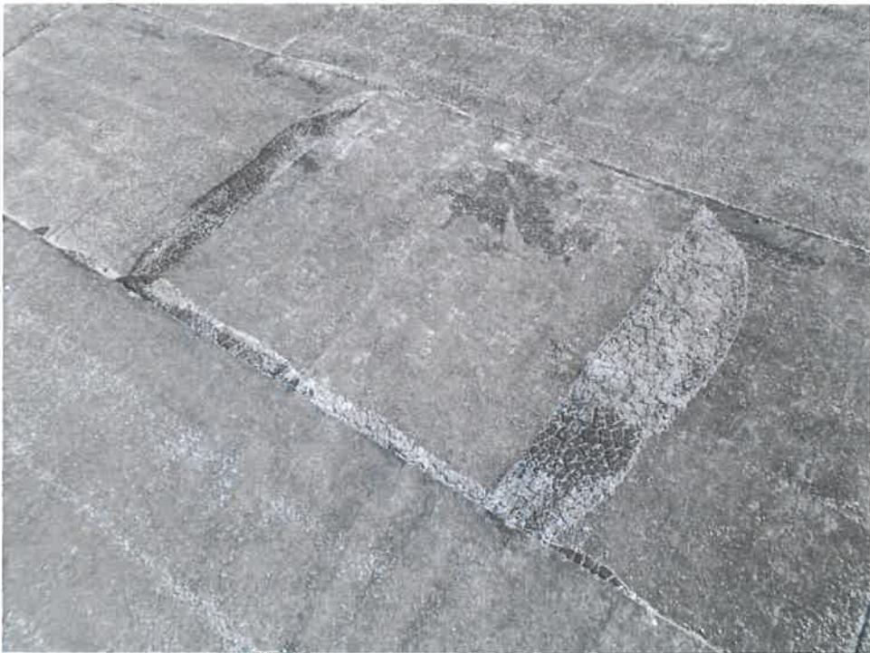
Figure 6: Extensive granule loss, deteriorated sealant, and patches are found on the north section of roof.
