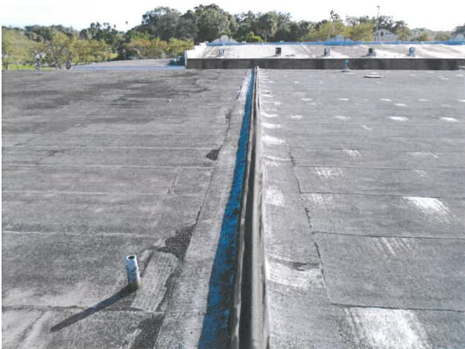
Figure 10: The expansion joint divides the north (left) section from the south (right) section of the roof.
