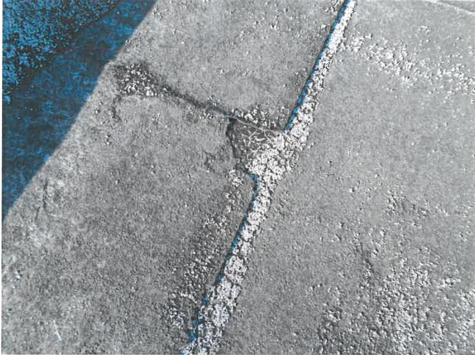
Figure 7: Deteriorated membrane and extensive granule loss are visible on the north section of roof.
