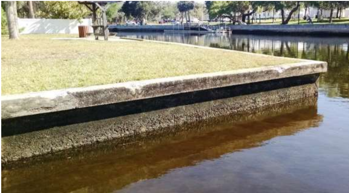
Figure 7 - Damaged Wall Caps
