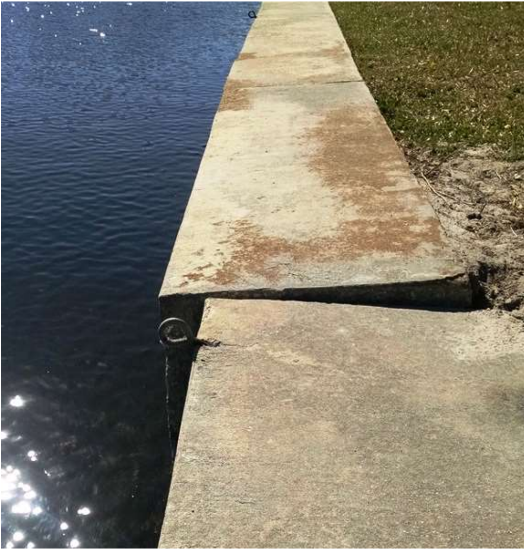
Figure 23 - Wall Leaning Toward River – Separation at Construction Joint (Looking South)
