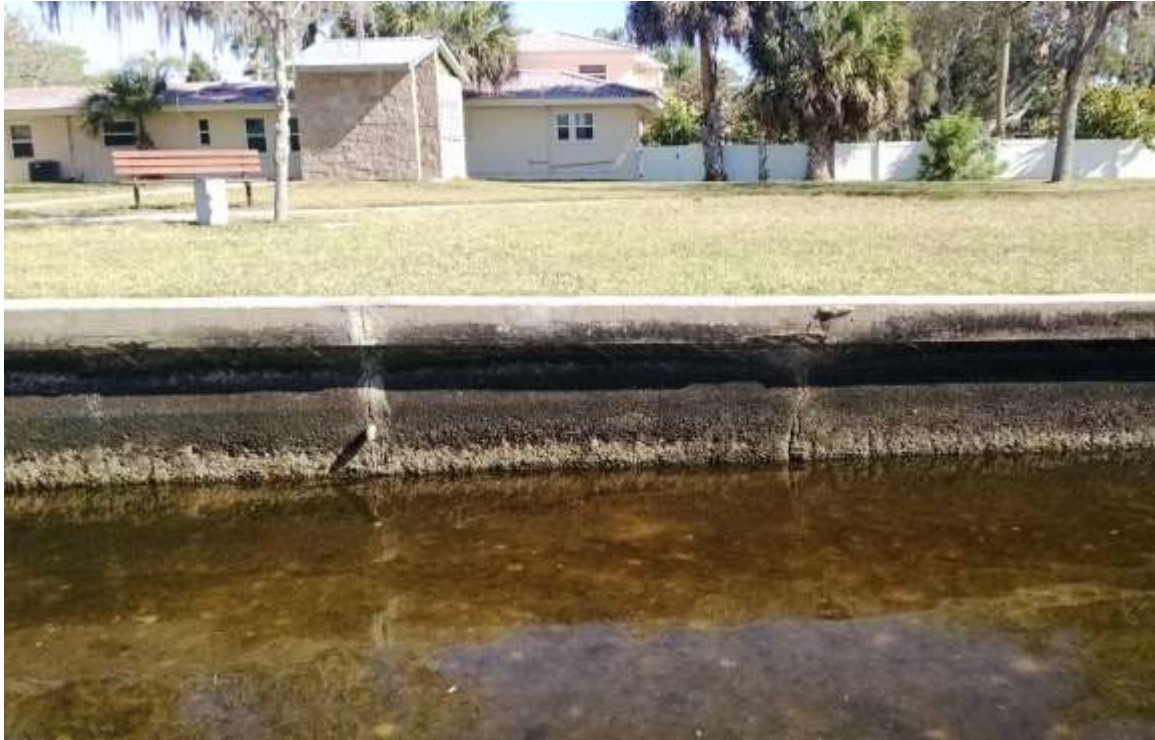
Figure 5 – Vertical Wall Crack
