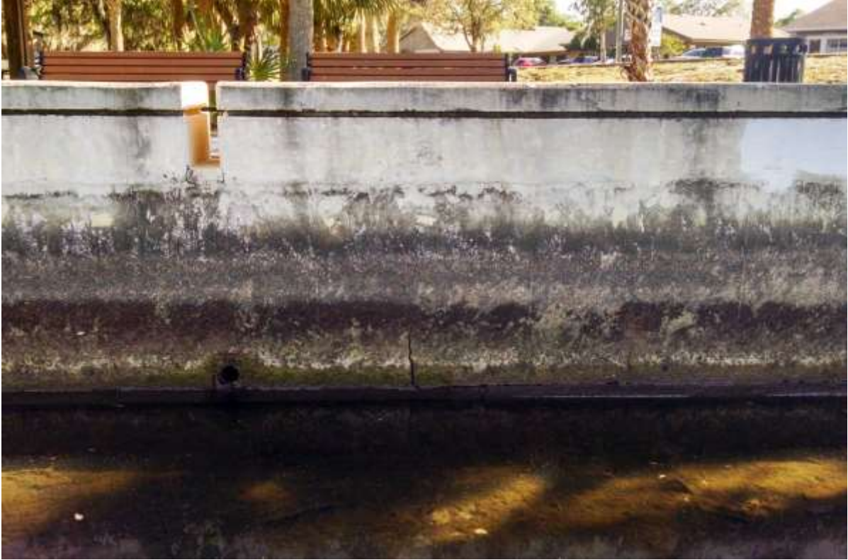
Figure 3 – Wall Crack at Base/Waterline
