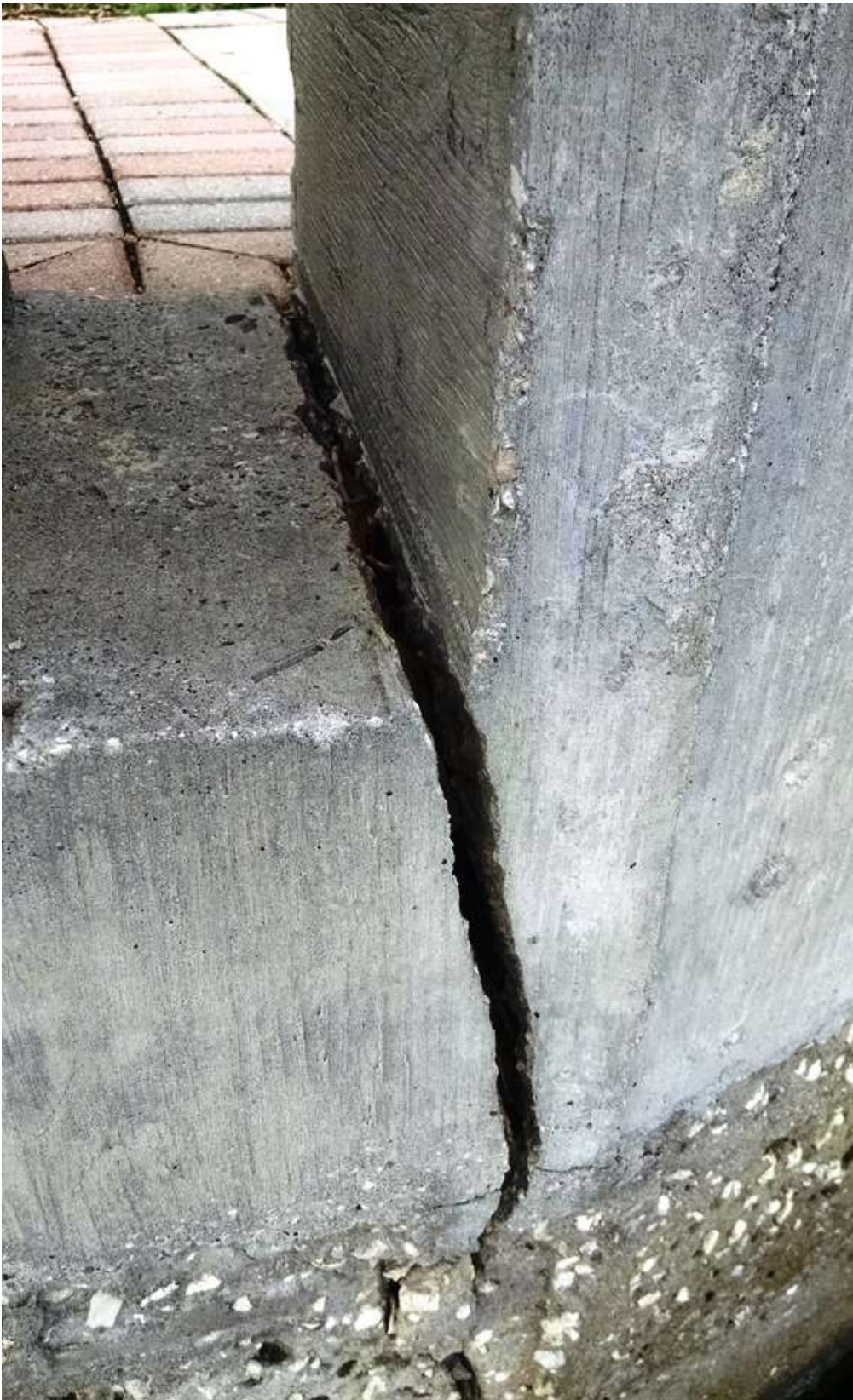
Figure 19 – Wall Crack at Spillway
