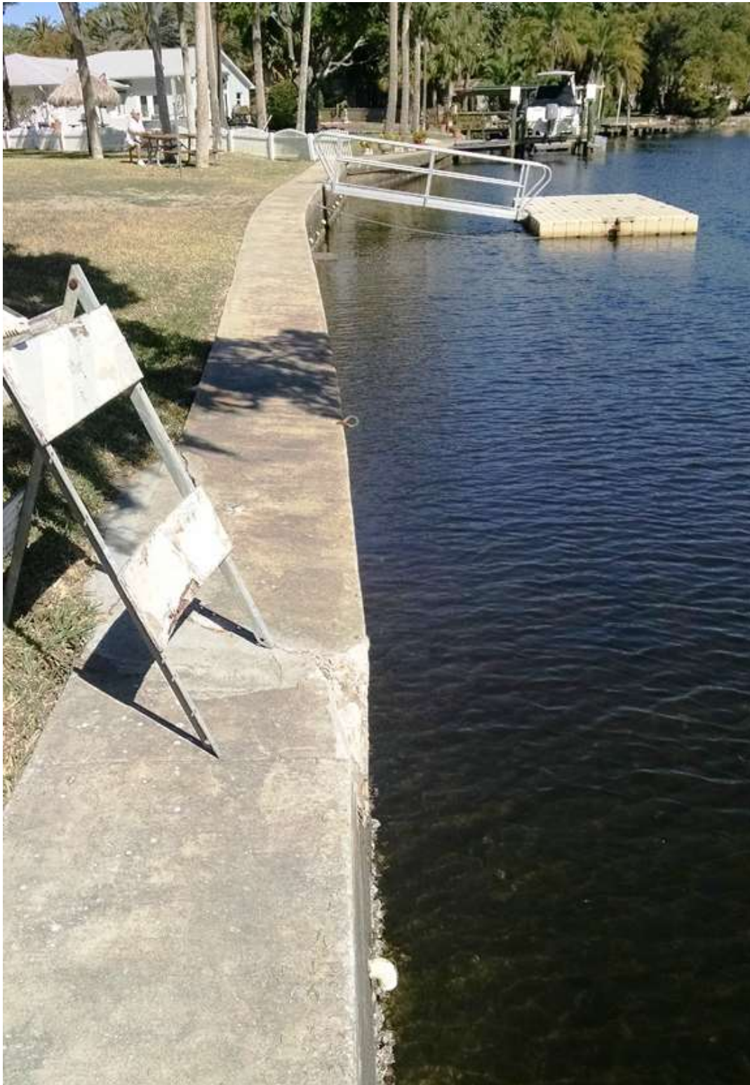
Figure 24 - Wall Leaning Toward River – Vertical Wall Crack (Looking North)
