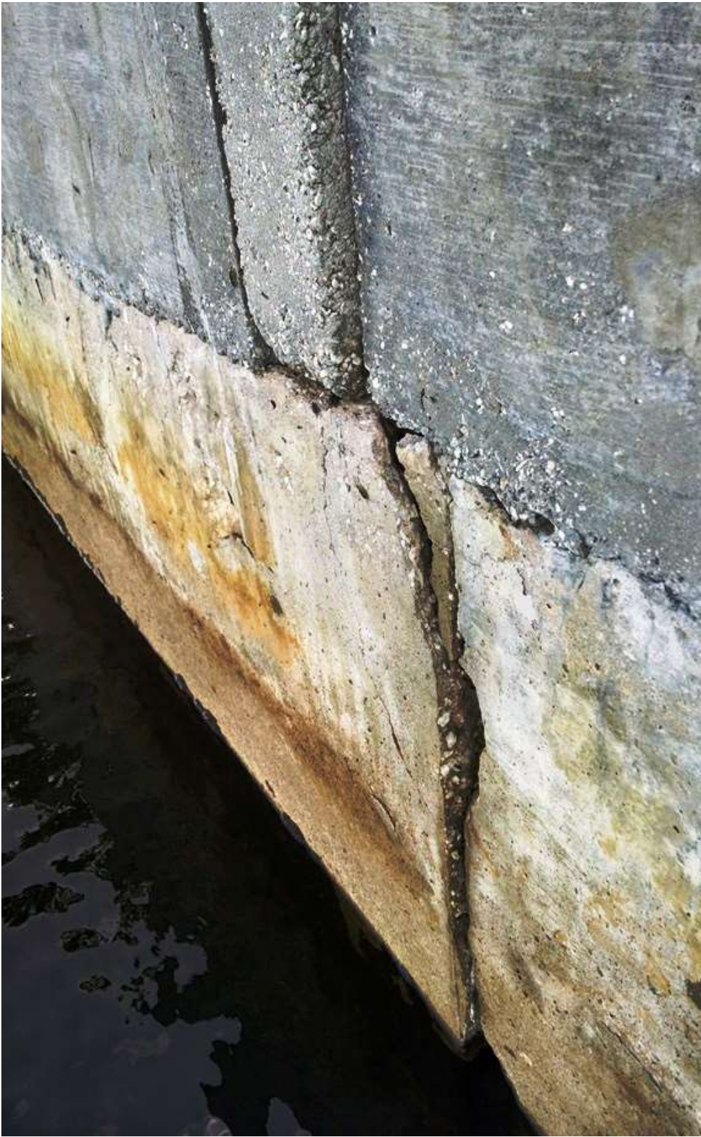
Figure 13 – Wall Crack/Shifting Outward
