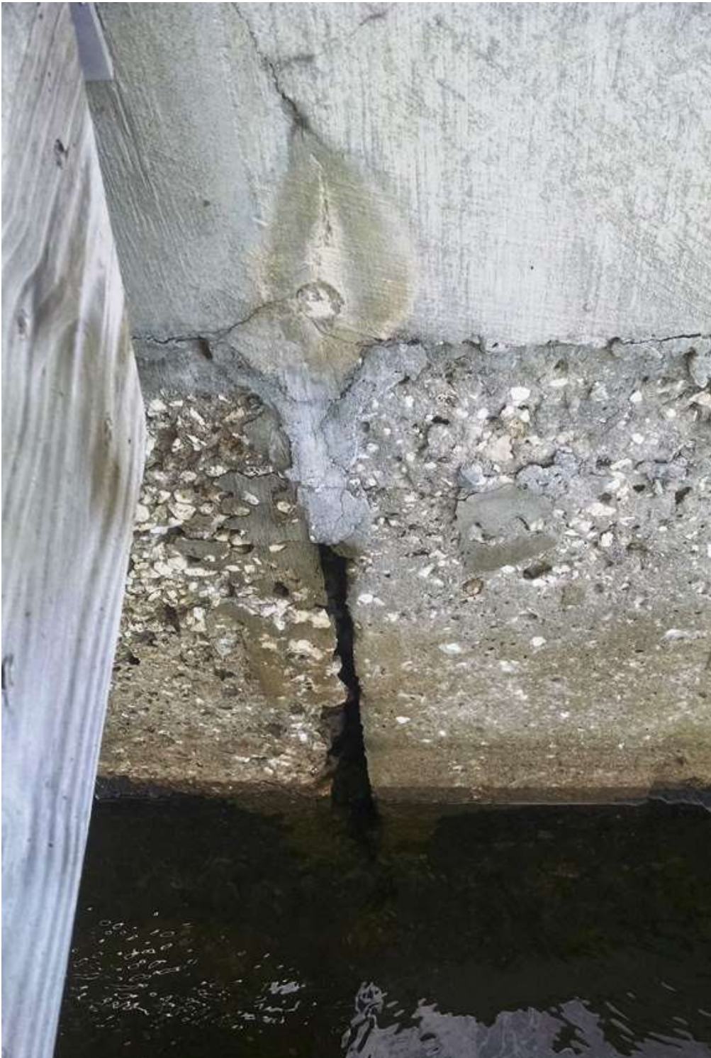
Figure 20 – Wall Joint Separation/Spalling
