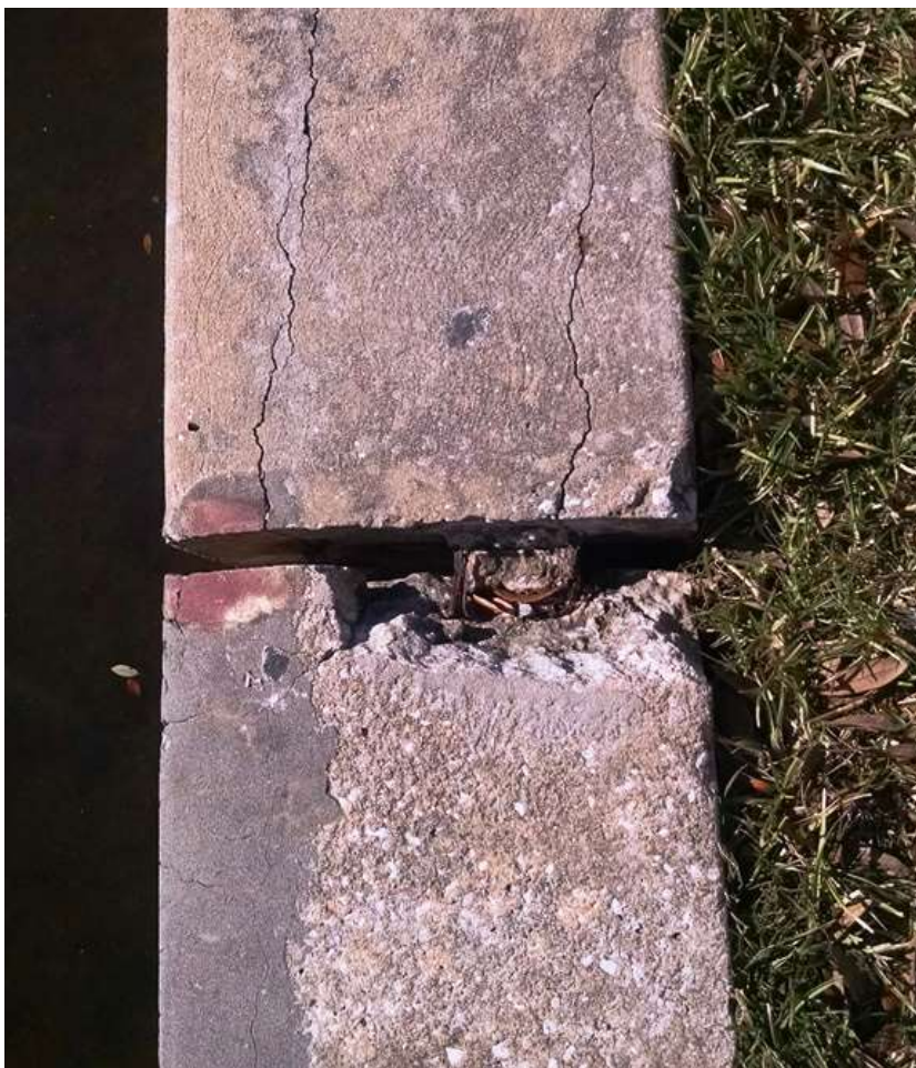
Figure 8 - Deterioration at Wall Joint
