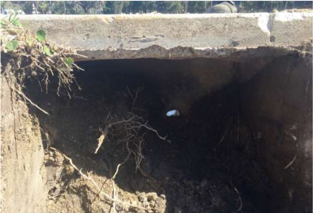
Figure 25 - Jasmine Park Seawall Drainage Hole Excavation – No Filter or Slotted Pipe Protection to Prevent Soil Erosion Through Hole
