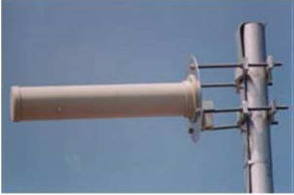
Exhibit 6. The antenna extends horizontally from the pole. This design is prohibited.
