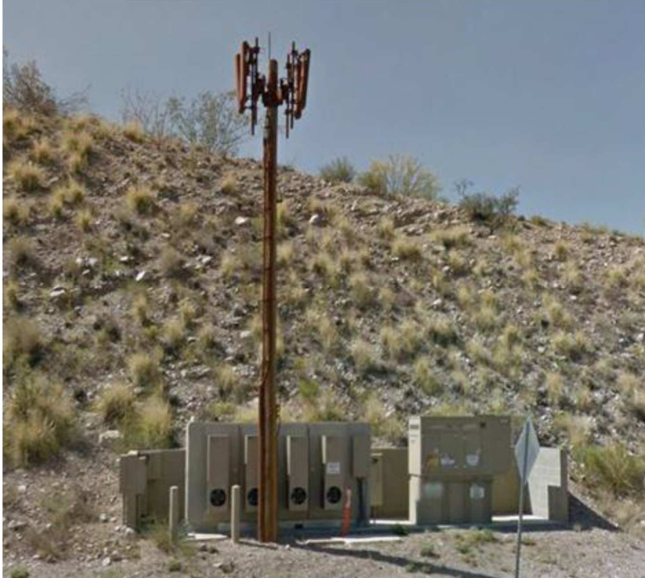
Exhibit 7. Antennas on arms are prohibited.
