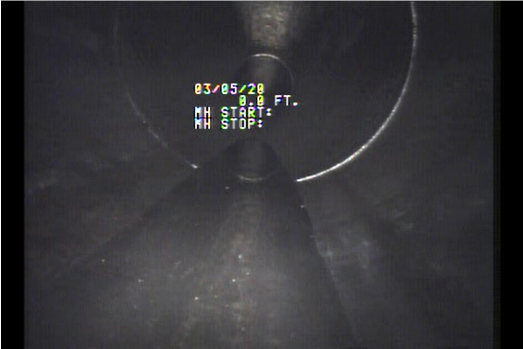
Figure B-1: CCTV Camera at Pipe Entrance of Oxidation Ditch #3.
