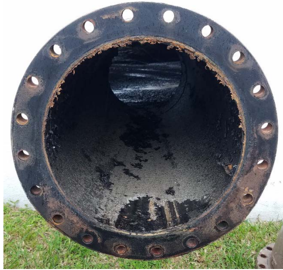
Figure 1-2: Exposed Interior of 24-inch Ductile Iron Gravity Main Pipe.
