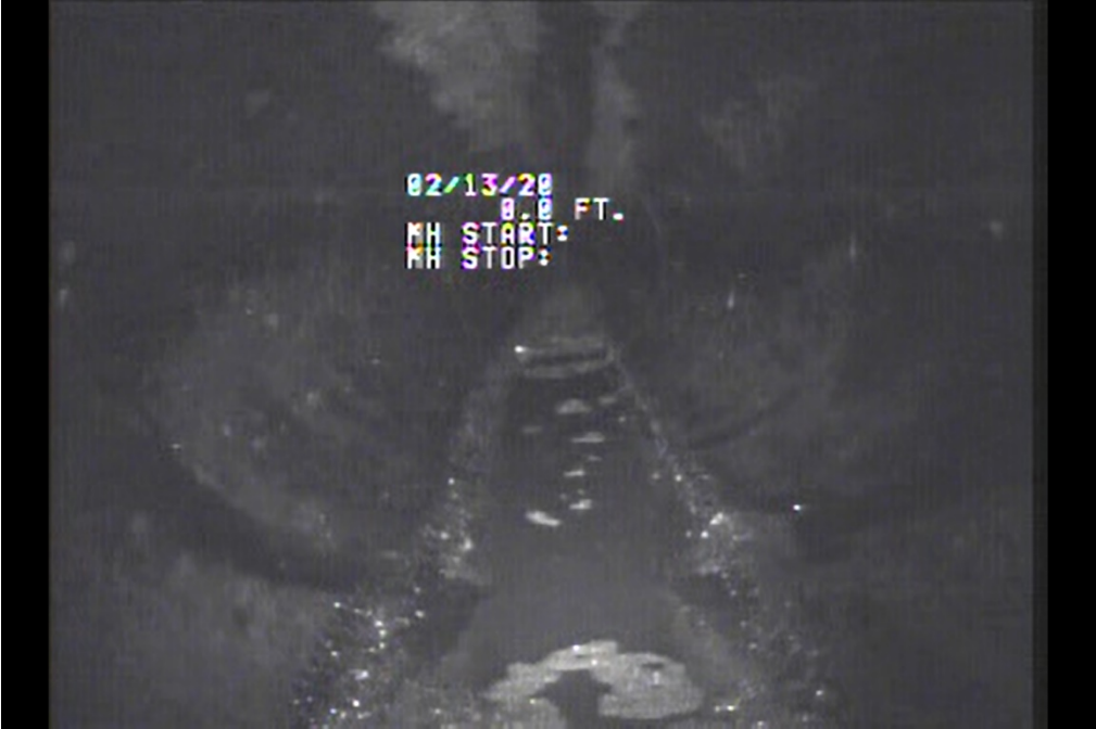
Figure B-6: CCTV Camera at Pipe Entrance of Oxidation Ditch #4.
