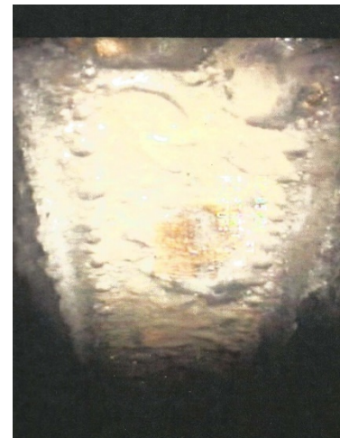
Figure 3-3: Interior Pipe Corrosion.
