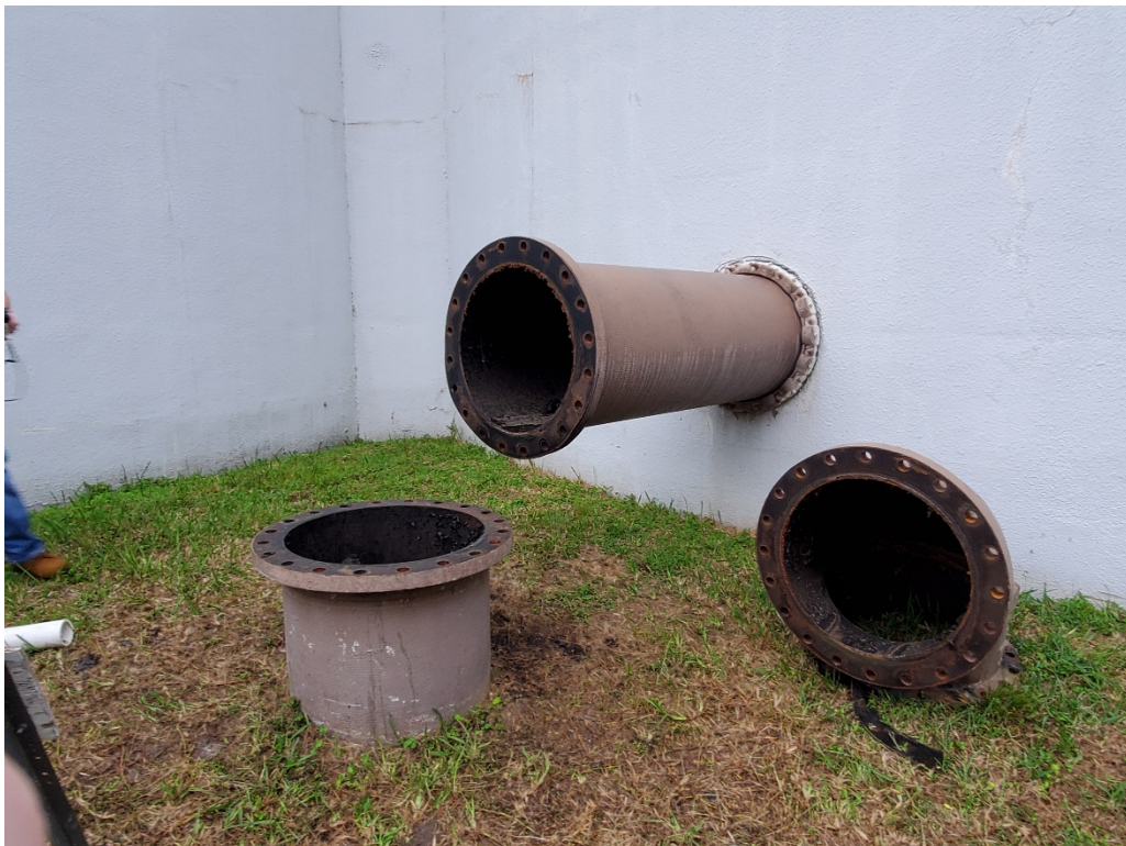
Figure C-2: Oxidation Ditch #4 Above-Grade Piping (UTT-2)
