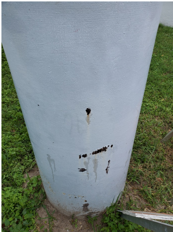
Figure C-8: Schreiber Plant Above-Grade Pipe Exterior Corrosion.
