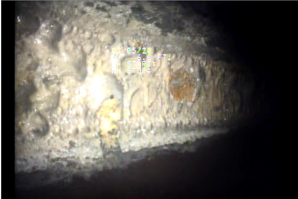
Figure B-3: Interior corrosion and 'caking' of solids.
