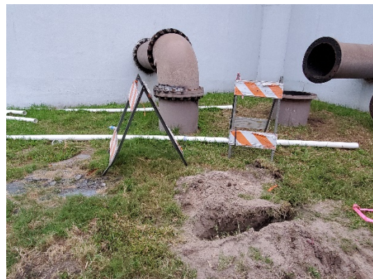
Figure 4-1: Oxidation Ditch Above-Grade Tank Piping.
