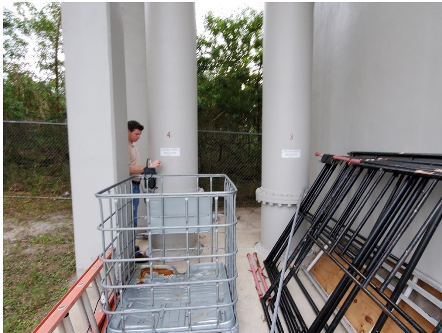
Figure C-6: Oxidation Ditch #3 and #4 Headwork Facility Piping (UTT-5, UTT-6)
