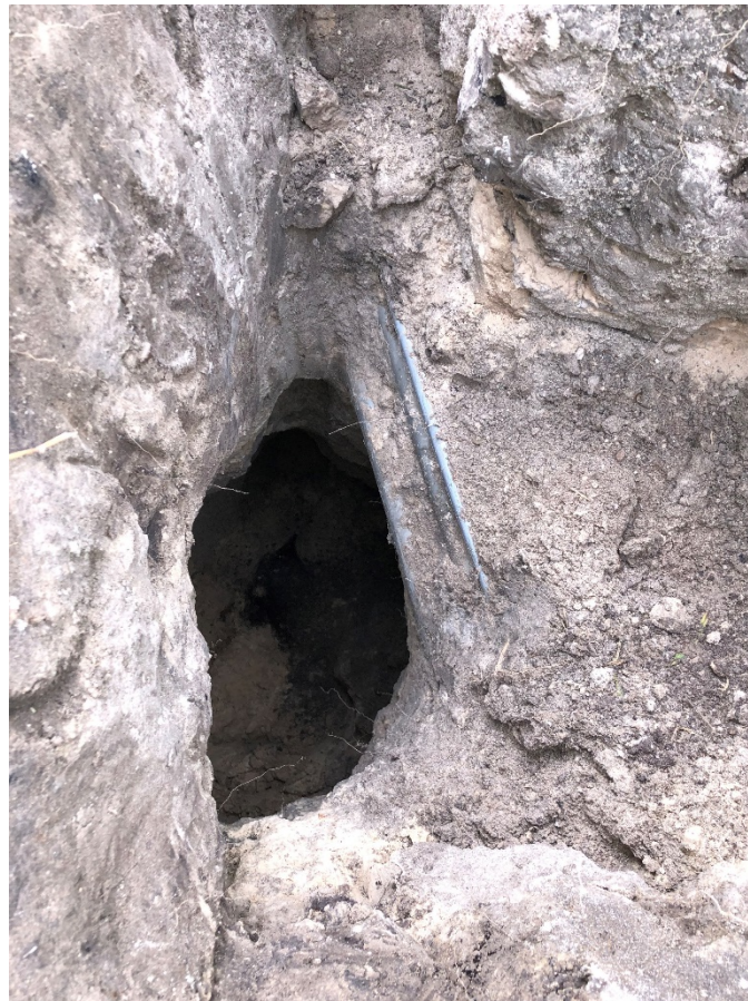
Figure C-10: Schreiber Plant Below-Grade Piping (UTT-8)
