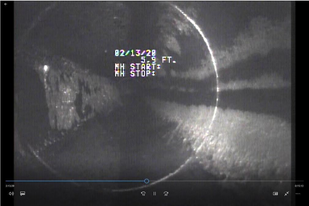
Figure B-8: White Film or 'Sheen' at Top and Bottom of Pipe (left and right).
