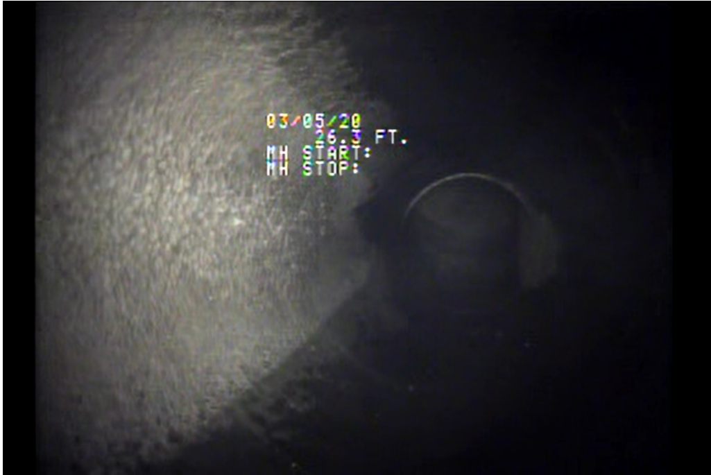
Figure B-5: White Film or 'Sheen' at Top of Pipe (left).
