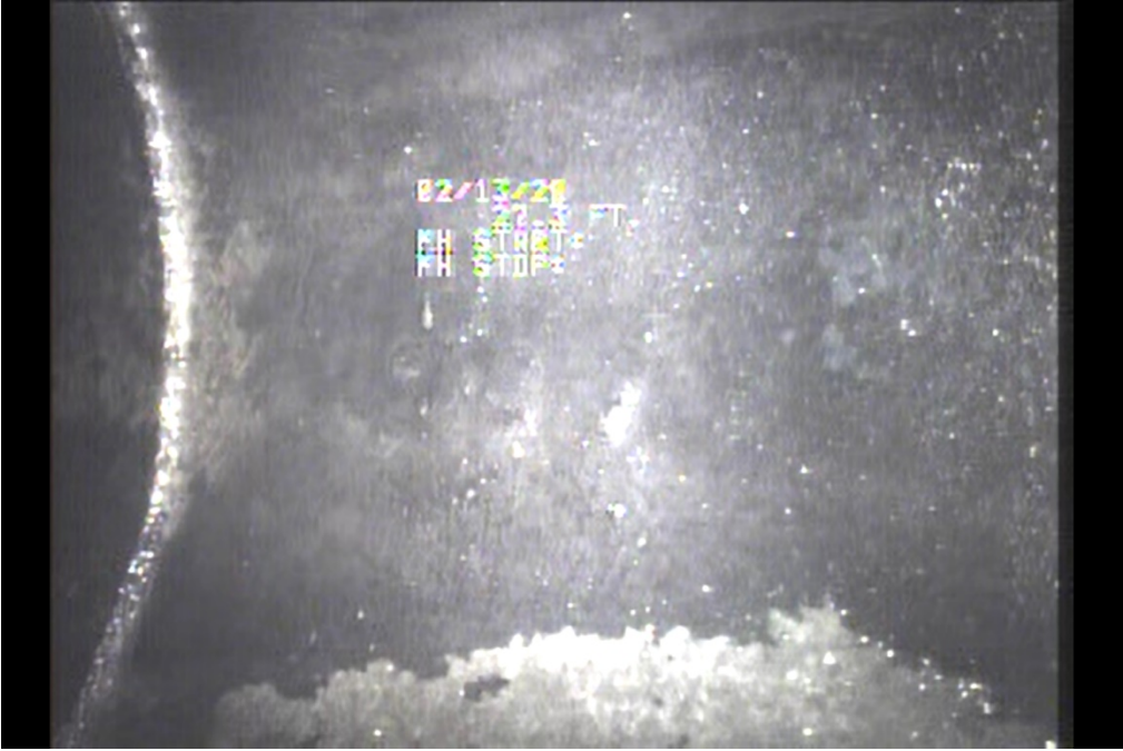
Figure B-10: Closeup of Impacts to Pipe Interior
