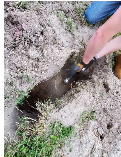
Figure 2-2: View of Exposed Pipe during UTT
