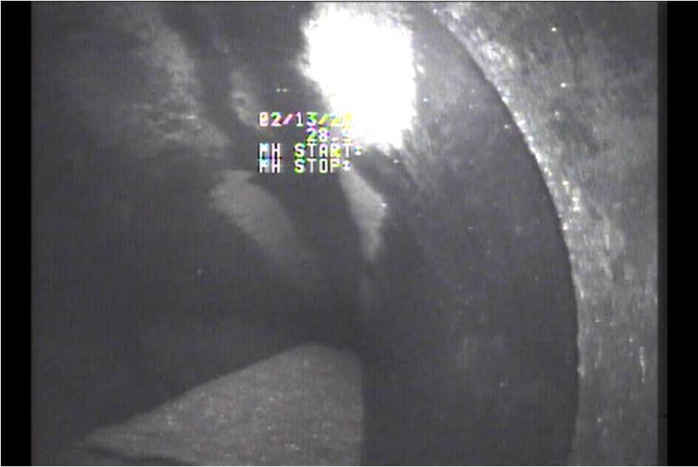
Figure B-11: Additional Pipe Wear Along Gravity Main.
