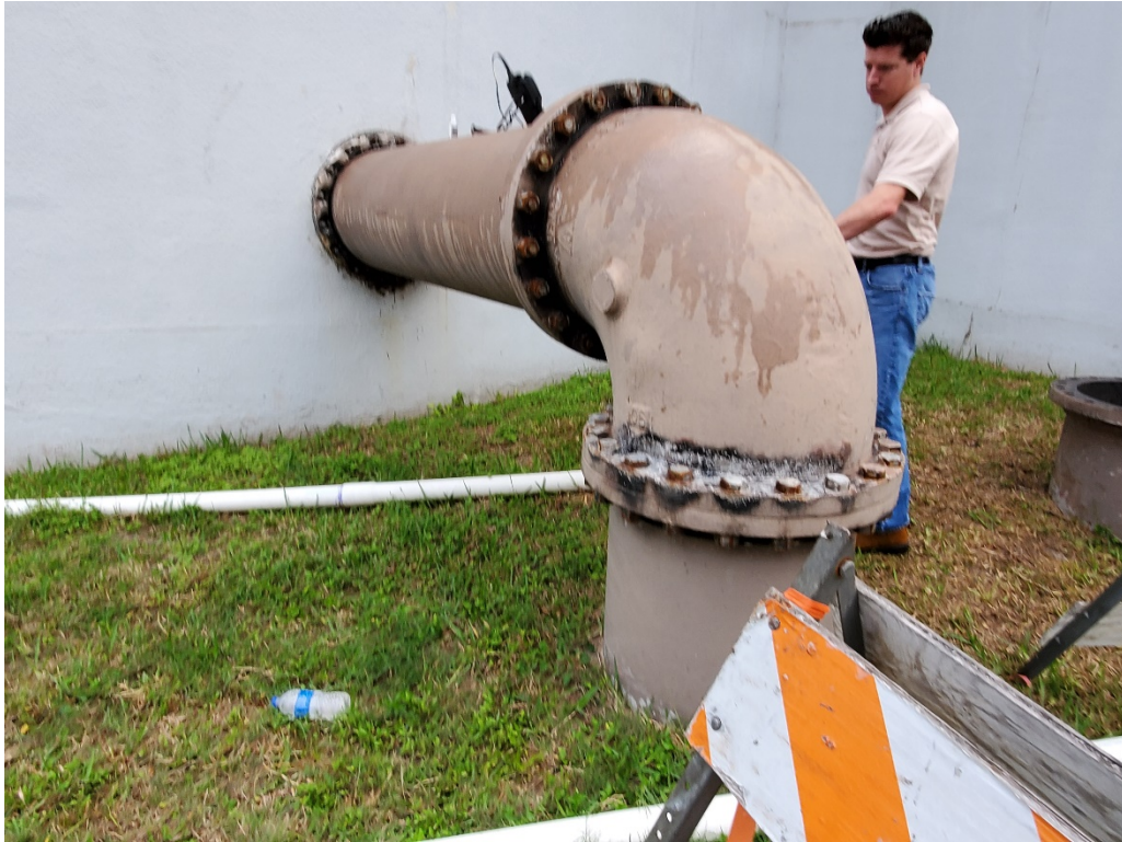
Figure C-1: Oxidation Ditch #3 Above-Grade Piping (UTT-1)
