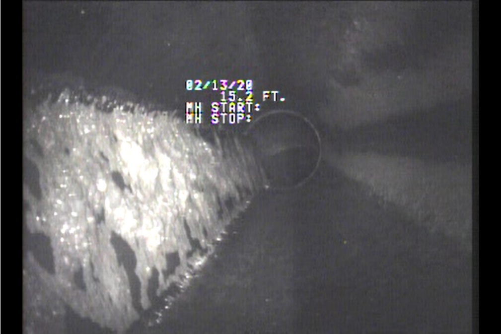
Figure B-9: Consistent White Film or 'Sheen' at Top and Bottom of Pipe (left and right).
