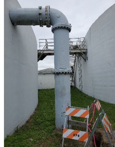
Figure 3-1: Schreiber Plant Piping.
