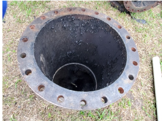
Figure 4-2: Interior Pipe Lining Deterioration.
