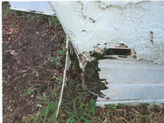
Broken piece of stucco on exterior
