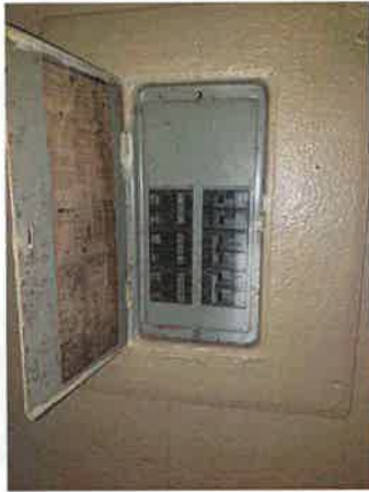
Breaker box located in living room
