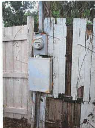
Electrical connection present
