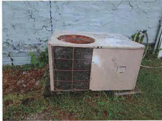
Central A/C unit, per owner, functional just disconnected
