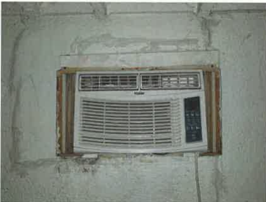
A/C unit in bedroom #3
