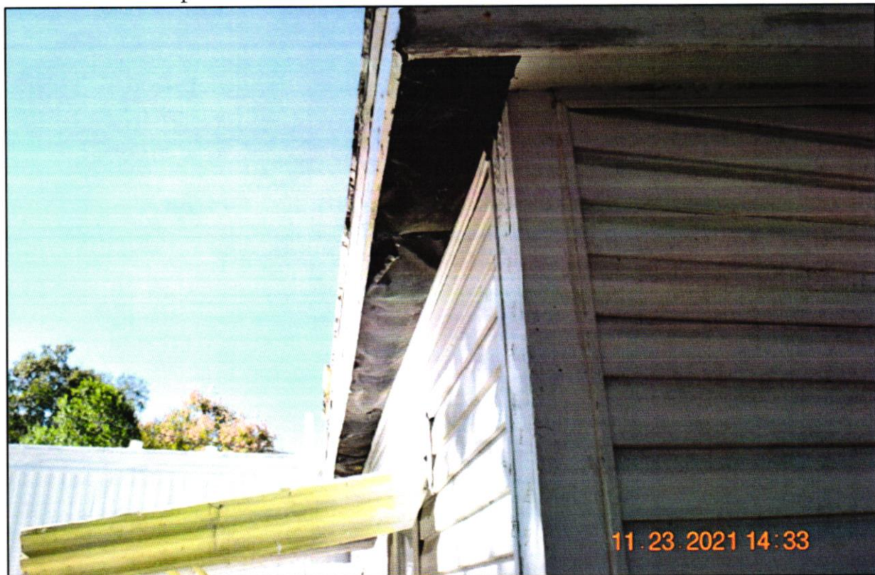
Shed - Soffits Unprotected from Rodents – Roof R-806.1
