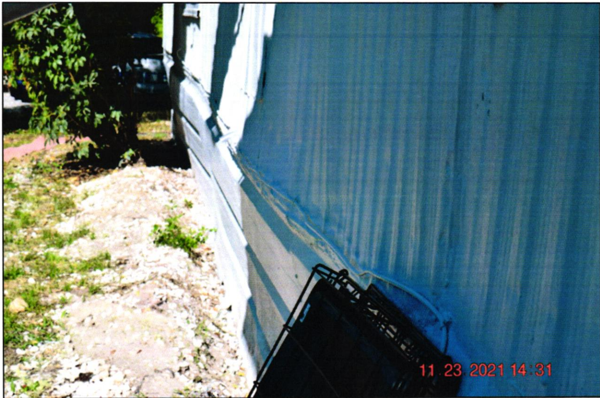
Mobile Home - Visual Sign of Falling Away of Siding
