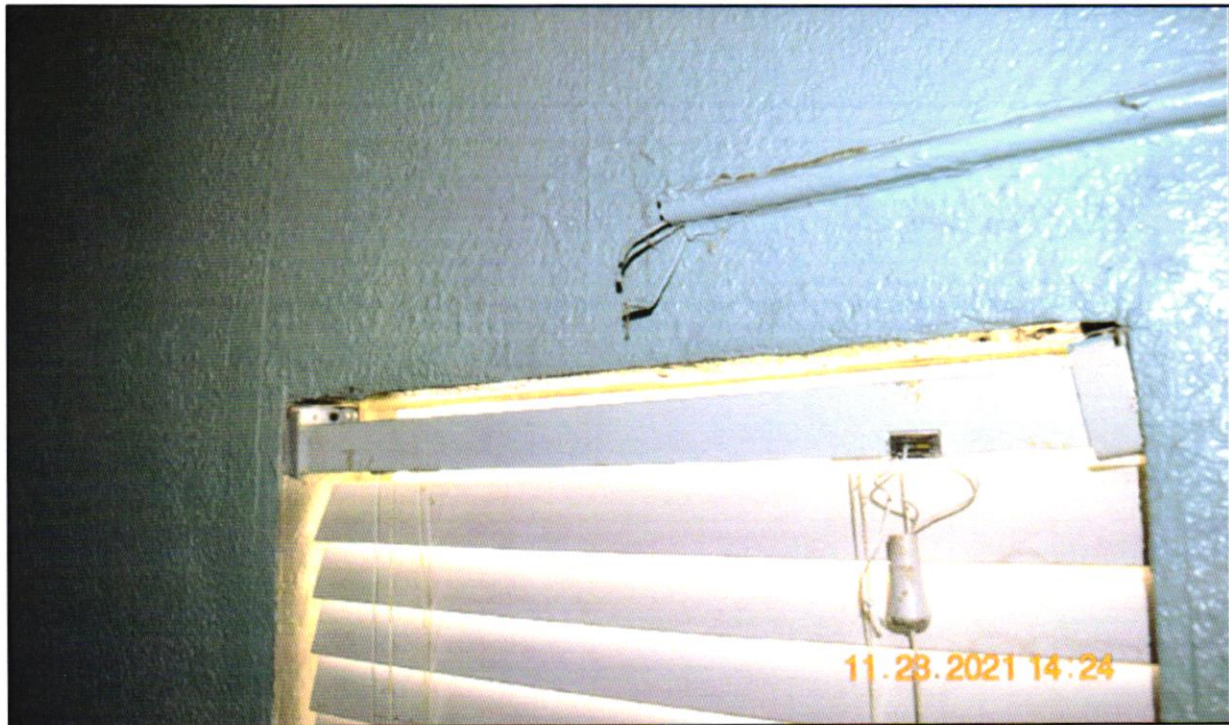
Shed - Unterminated Electric Conductors – National Electrical Code 110.24
