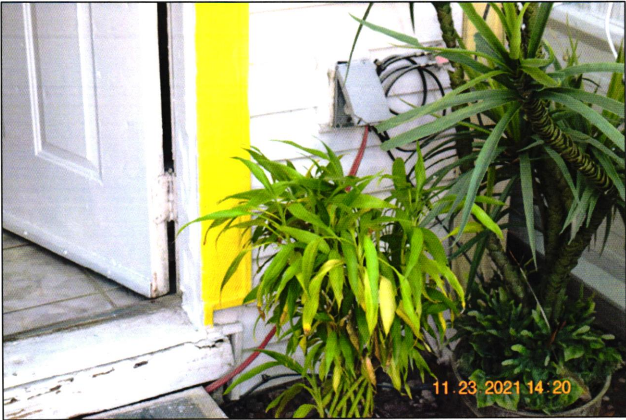
Shed - Unprotected Romex Wire – National Electrical Code 334.12
