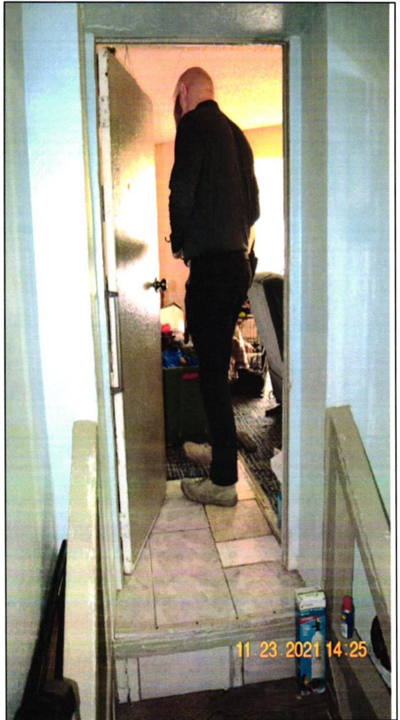
Unpermitted Secondary Entrance into Prefab Mobile Home Florida Administrative Code 61-41.011
