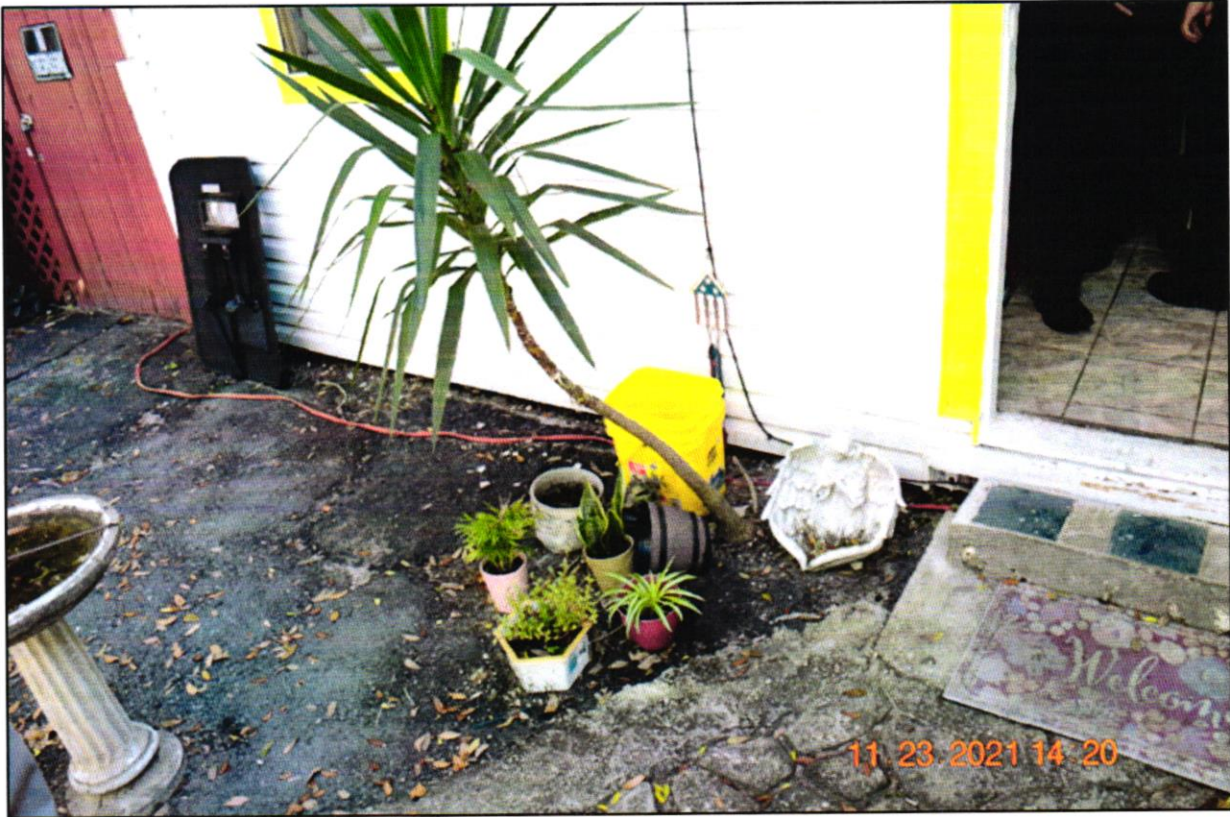
Shed - Unprotected Romex Wire – National Electrical Code 334.12
