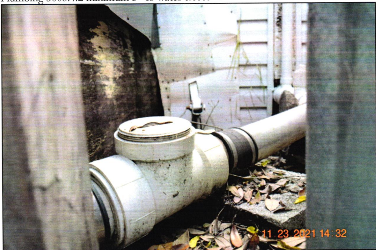
Pipe Undersized for Restroom Plumbing 3005.1.6 reduction in size Plumbing 3005.4.2 minimum 3" to water closet
