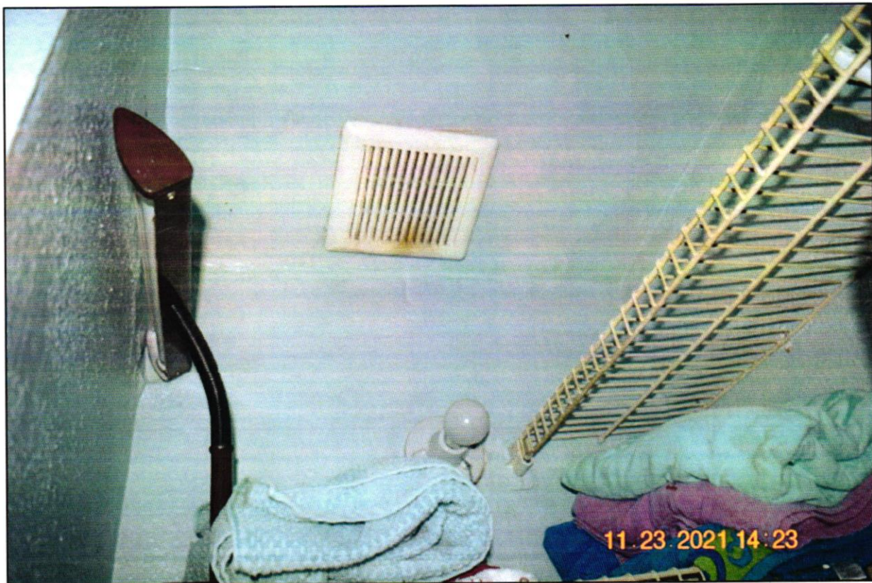
Shed - Unprotected Light Fixture in Closet - National Electrical Code 1410.97 and 410.16
