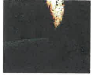
PHOTO OF RUSTED COLUMN AT STAIRS SCALE: 1/8" = 1'-0"
