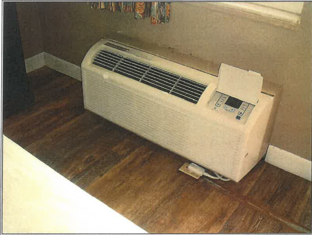
Typical AC and Heat Unit
