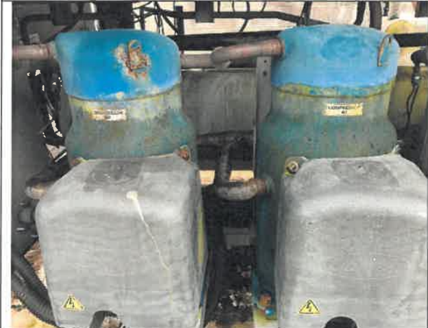
Photo 5 – Original Compressor A1 & A2
