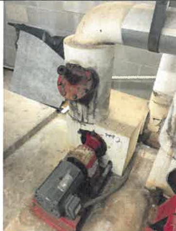
Photo 4 – Existing Chilled Water Pump #2
