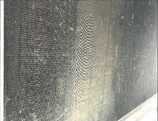
Photo 7 – Existing Chiller Fins
