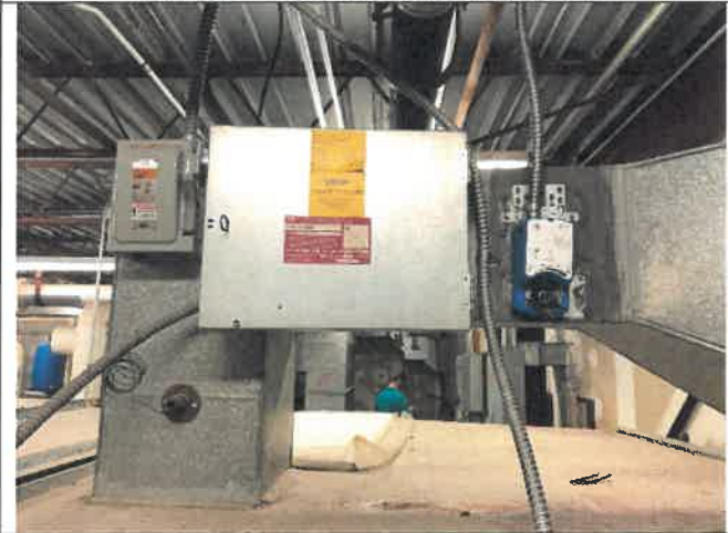
Photo 11 – Electric Duct Heater
