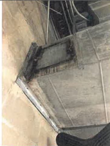
Photo 11 – Leaking Duct Seams
