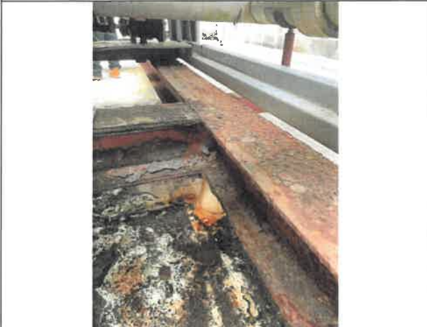
Photo 13 – Deteriorated Chiller Support
