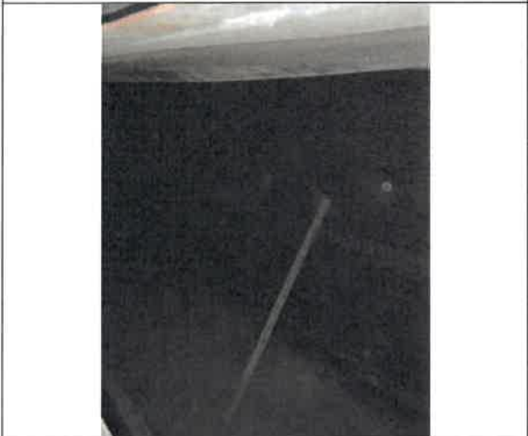
Photo 7 – Internally Lined Ductwork
