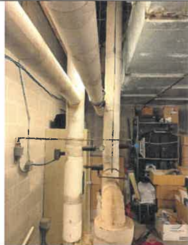
Photo 12 – Existing Pneumatic Controls
