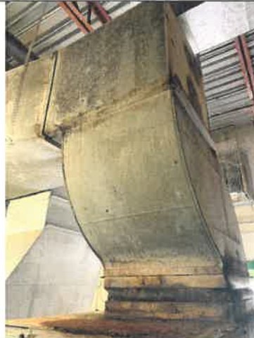
Photo 8 – Leaking Duct Seams
