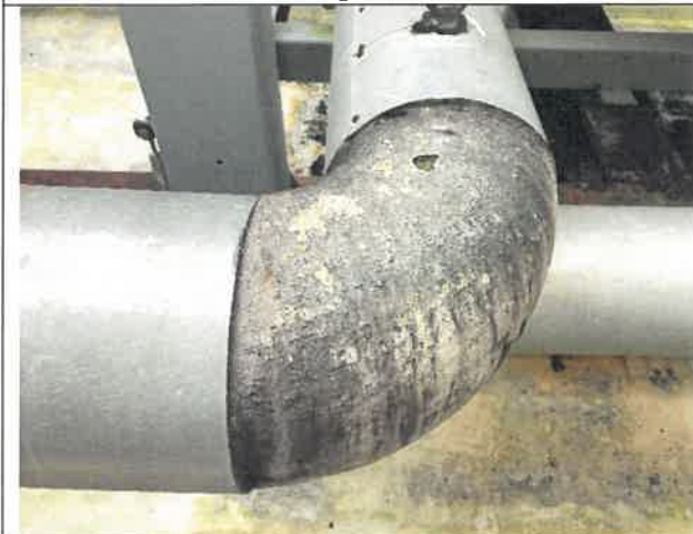
Photo 11 – Missing CHWP Jacketing
