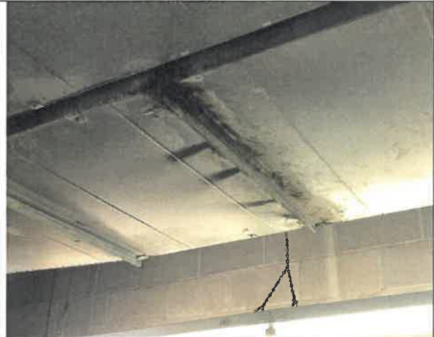
Photo 14 – Leaking Duct Seam
