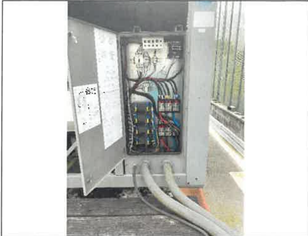
Photo 3 – Existing Chiller Controls
