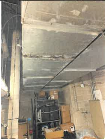
Photo 13 – Leaking Duct Seams
