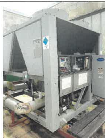
Photo 2 – Existing Chiller Controls
