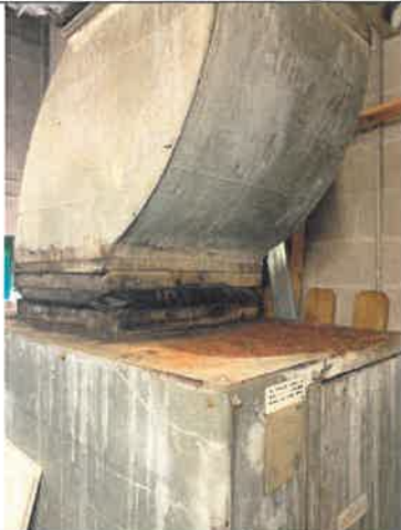
Photo 7 – Leaking Duct Seams
