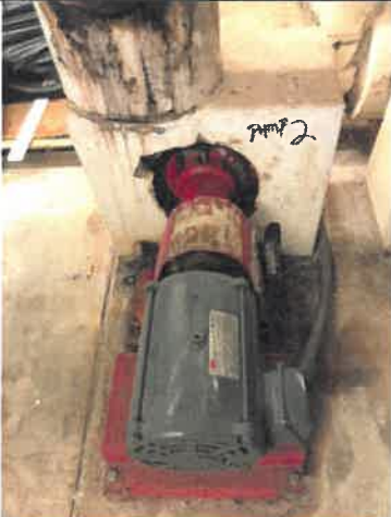
Photo 3 – Existing Chilled Water Pump #2
