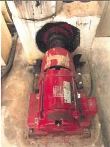
Photo 1 – Existing Chilled Water Pump #1
