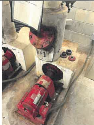
Photo 2 – Existing Chilled Water Pump #1
