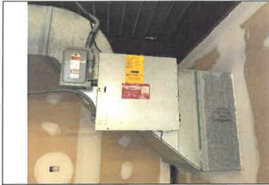
Photo 9 – Electric Duct Heater
