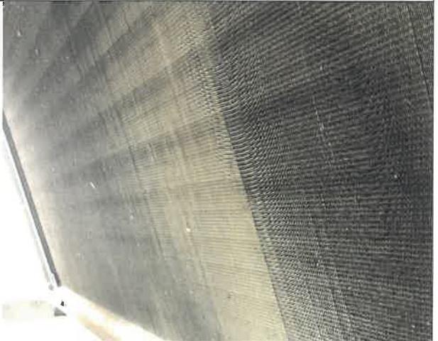
Photo 8 – Existing Chiller Fins
