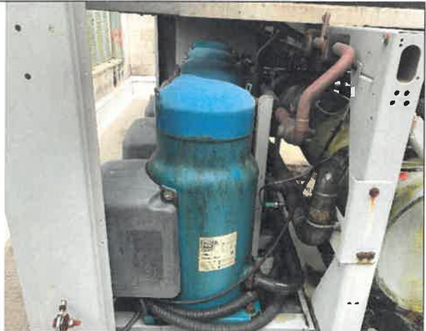
Photo 4 – Compressor Bank and Piping
